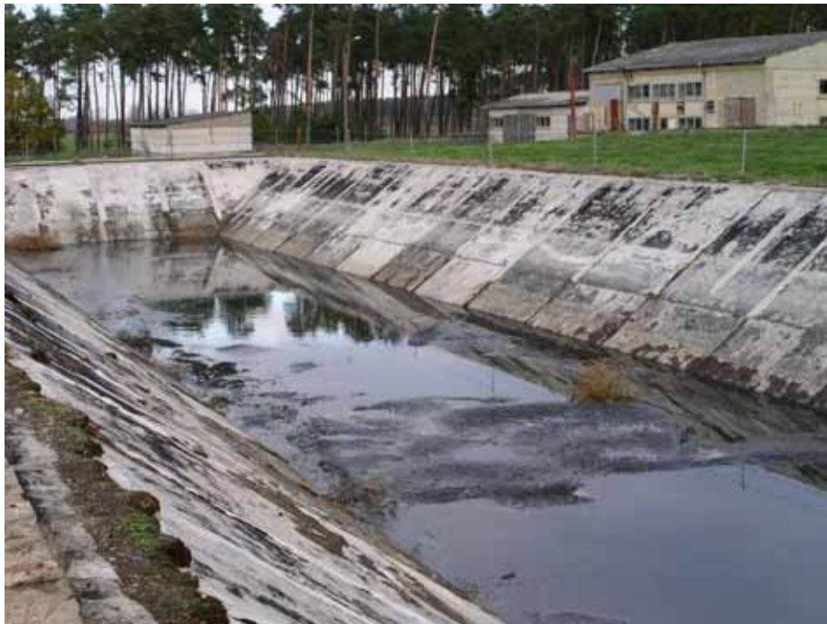
Fig. 2 One of eight lagoons where pig manure is stored resulting in appr. 670 tons methane emissions annually (14.100 t CO 2 e/a)
